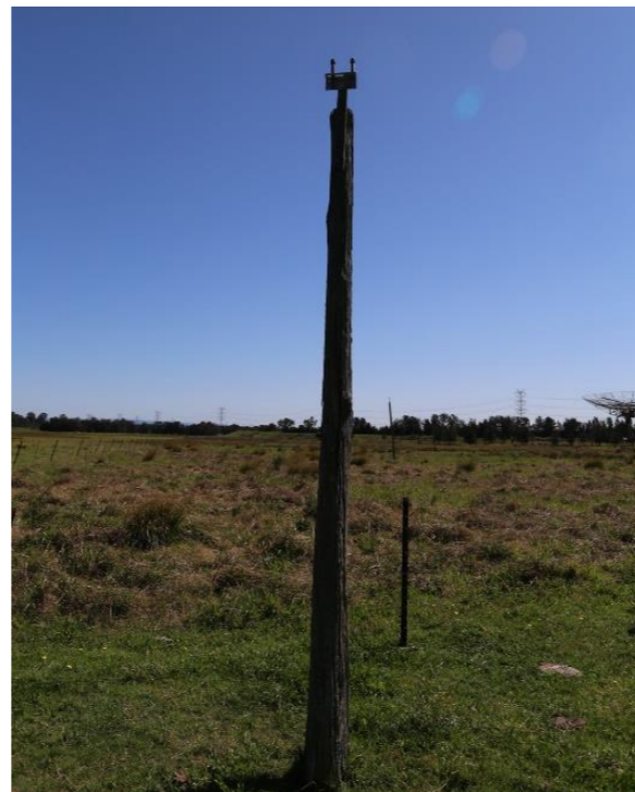
Figure 19. Remnant pole at Fleurs. The original installation would have involved hundreds of these poles in a straight row. They would have supported various wires and insulators relating to the Shain Cross. Source: Extent Heritage.
