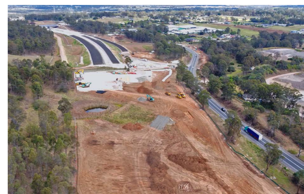
Earthworks on the southern side of Elizabeth Drive between Tank Road and Cecil Road
