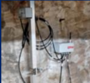
An underground monitor in a basement
