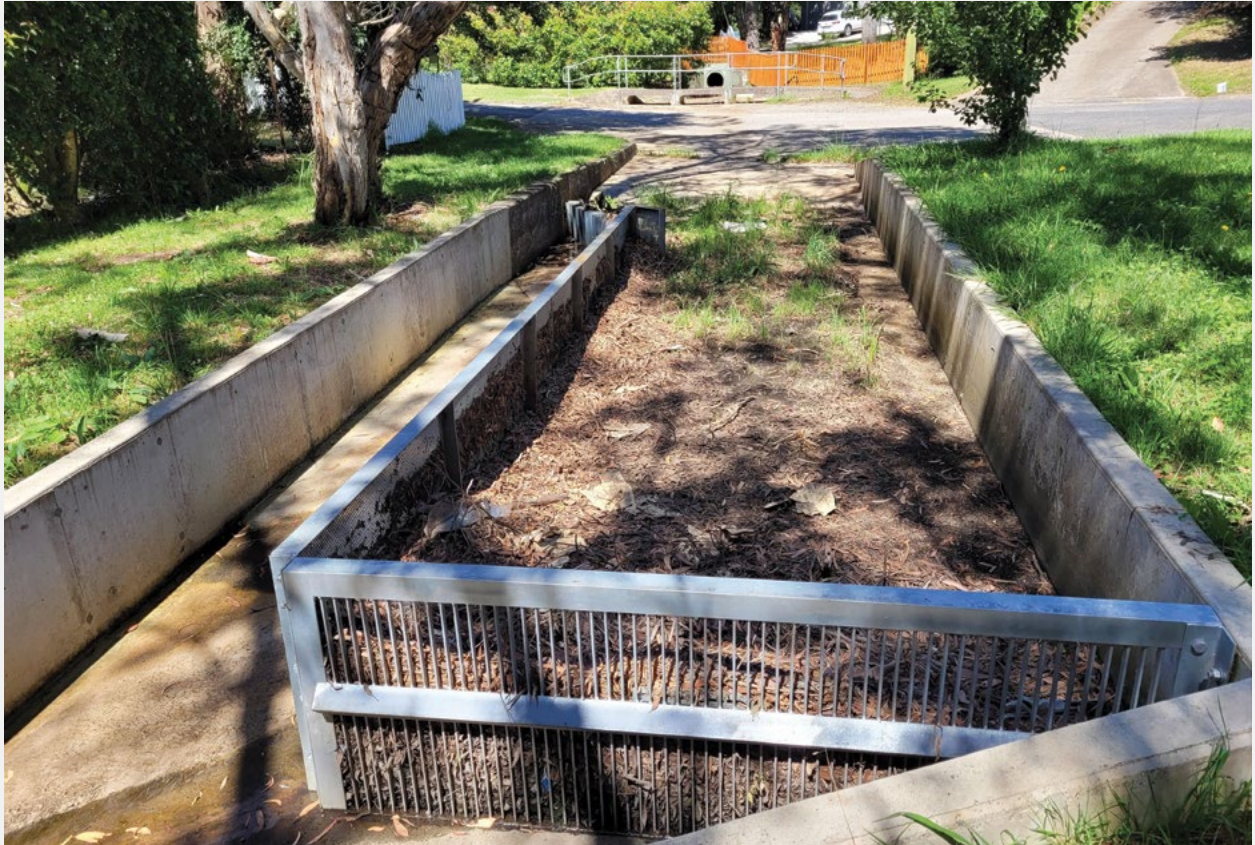
Rain gardens like those installed by Blue Mountains City Council will be used to filter stormwater
