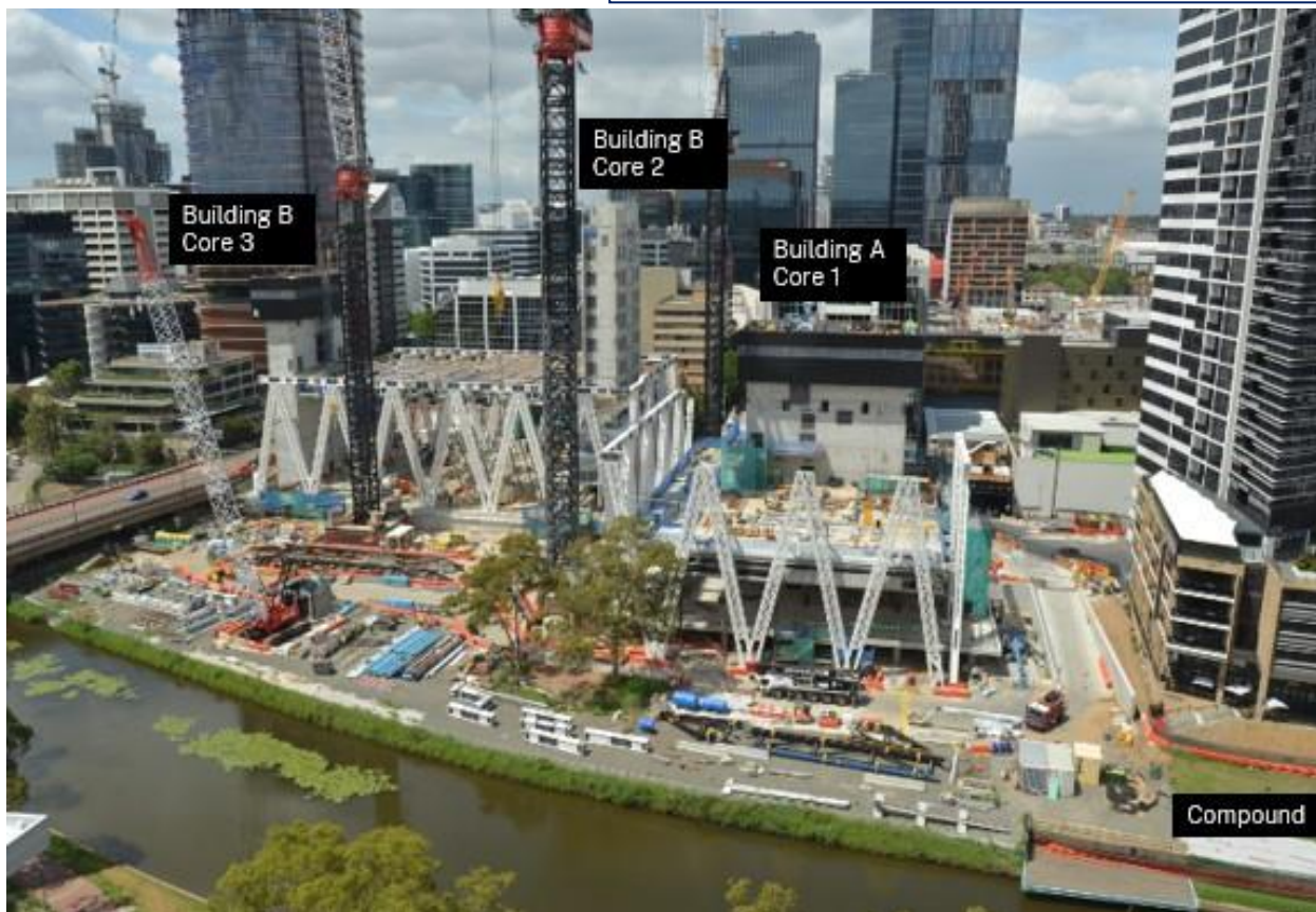
Image: Powerhouse Parramatta construction site, with new compound established; credit: Images for Business
