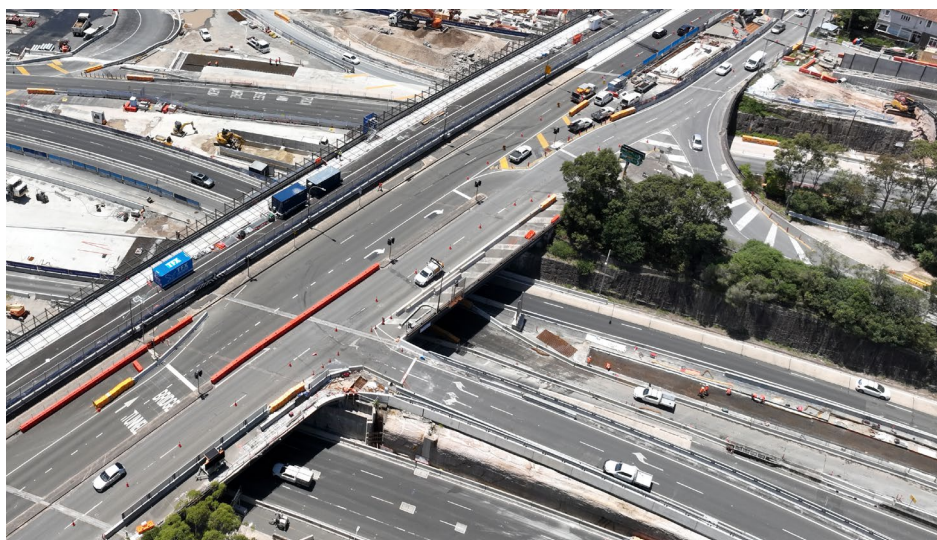
Aerial view of Ernest Street shared user bridge works taken in January 2025.
