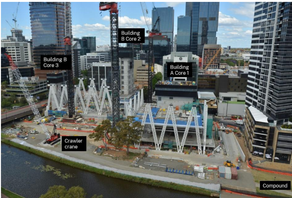
Image: Powerhouse Parramatta construction site, with new compound established; credit: Images for Business
