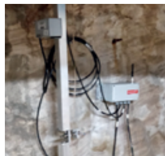
An underground monitor in a basement
