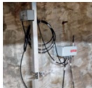
An underground monitor in a basement
