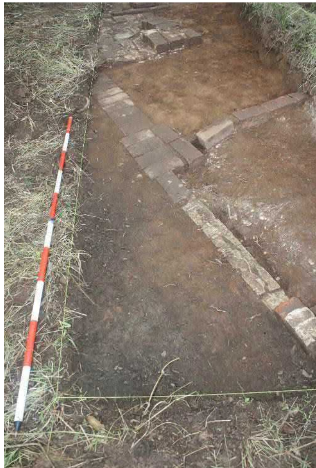
Figure 5-7 Test Trench 1, north-east corner showing the service trench [ and possible yard surface [C015].
