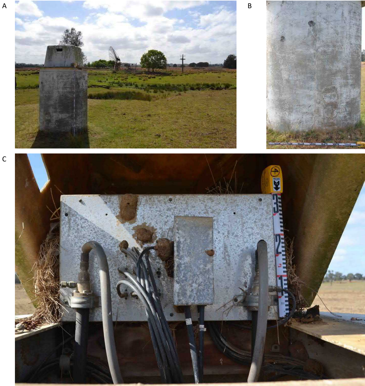
Figure 19 South Creek 1 Antenna Complex signal box. A: box looking east. B: possible service openings C: cable harness inside signal box.
