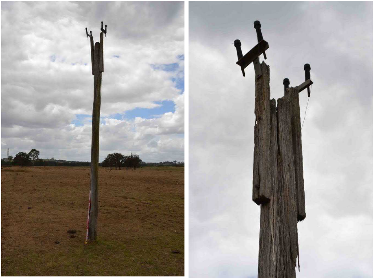
Figure 34 Shain Cross SC01: (left) general view; (right) detailed view.
