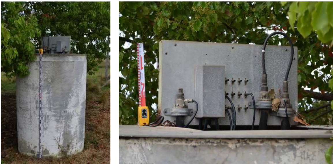
Figure 27 South Creek 2 Antenna Complex: signal box.
