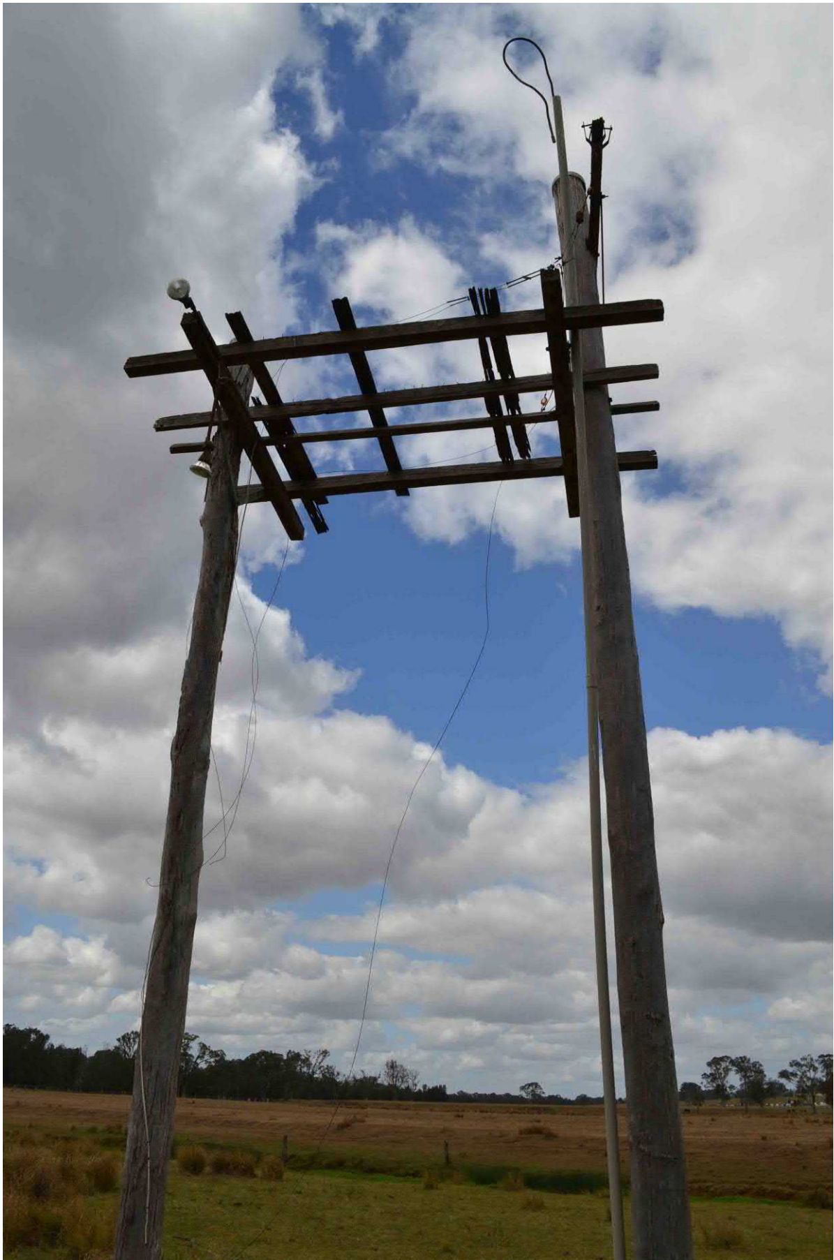
Figure 28 South Creek 2 Antenna Complex: power structure.
