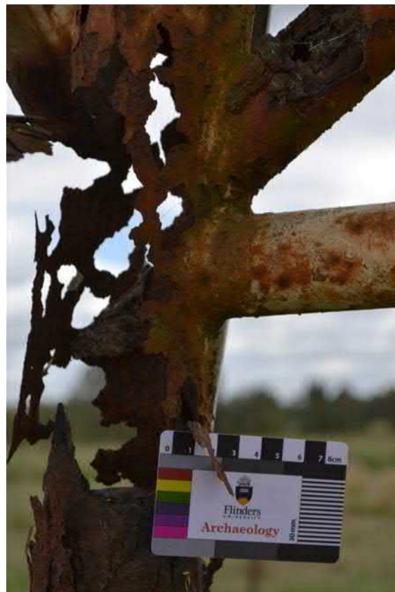
Figure 32 North Antenna showing an area of severe rust damage.
