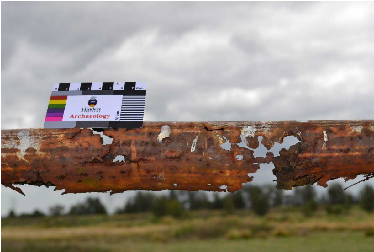
Figure 31 North Antenna showing rust damage.
