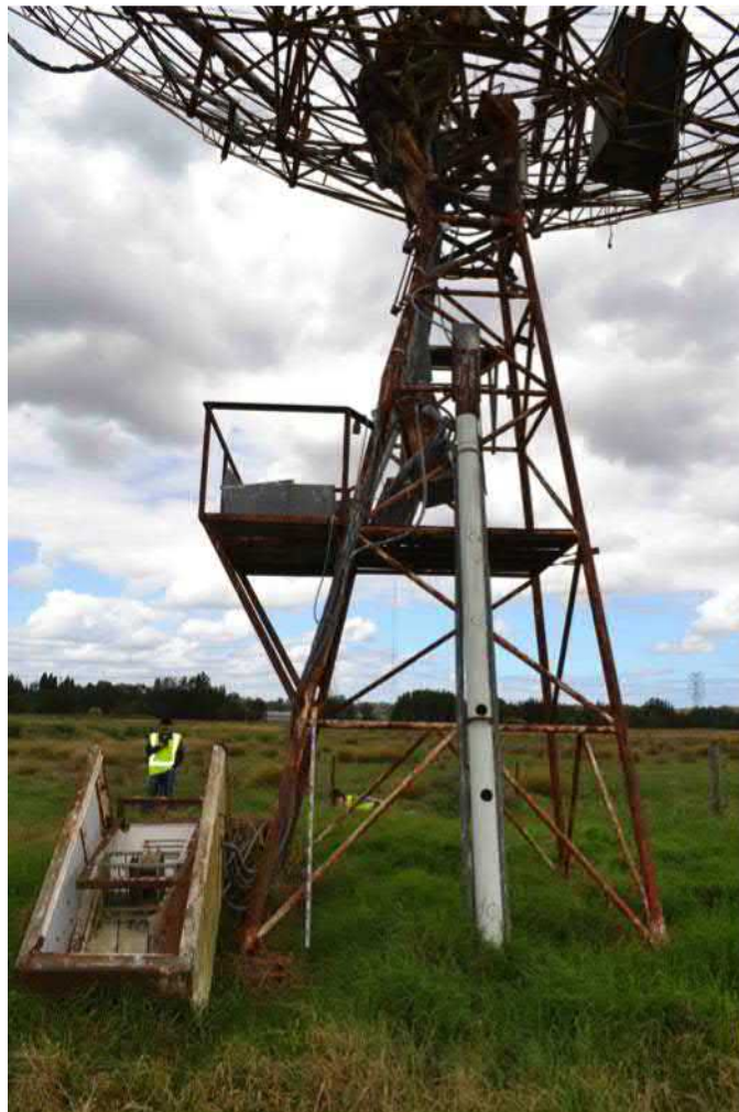
Figure 29 North Antenna showing fallen signal box.
