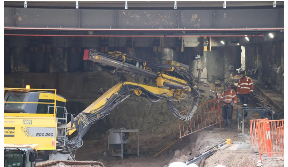
Excavation of the cut and cover decline at the Ridge Street construction site
