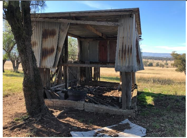
Plate 4: Dilapidated timber and metal shed (photo AECOM)
