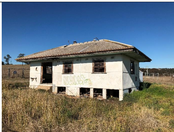
Plate 1: Abandoned house fenced due to asbestos (photo AECOM)
