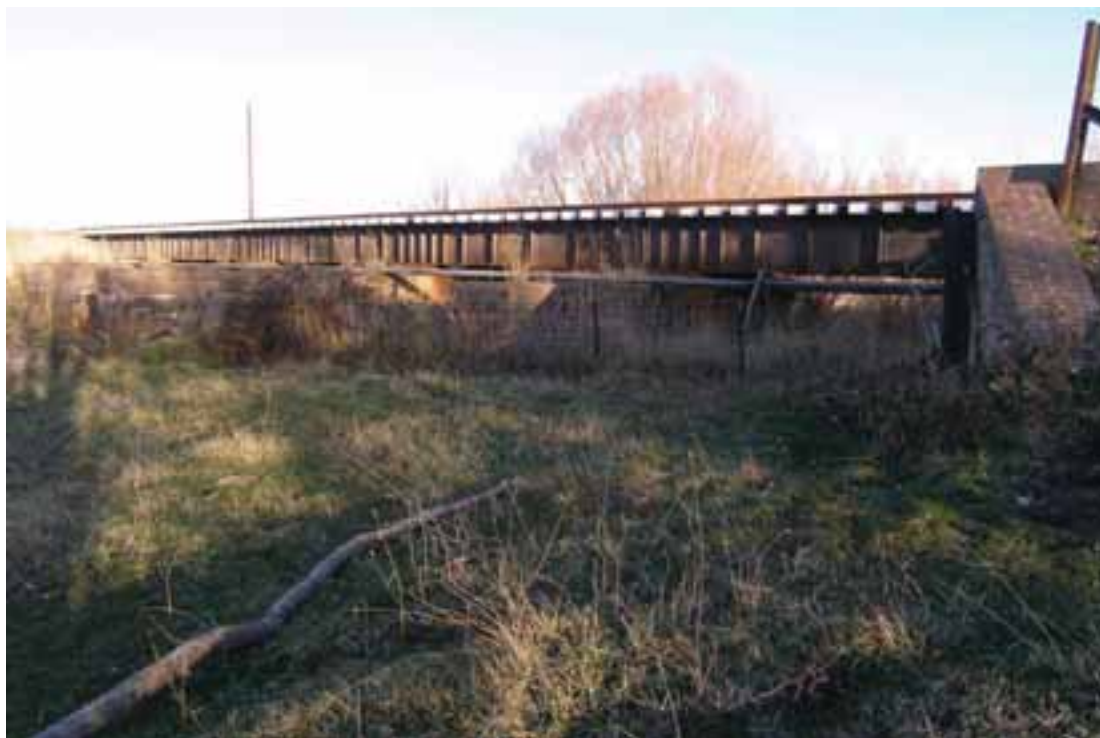
Plate L3-3. Railway bridge, over Belubula River, 400 metres east of Blayney Railway Station, Blayney, looking south-east.
