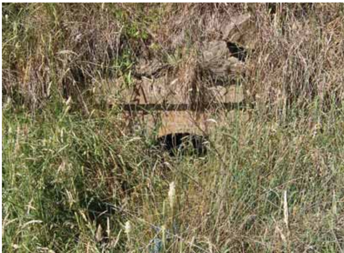
Plate L3-4. Railway culvert, with brick arch, at north-west corner of site for proposed CVO Dewatering Facility, Blayney.
