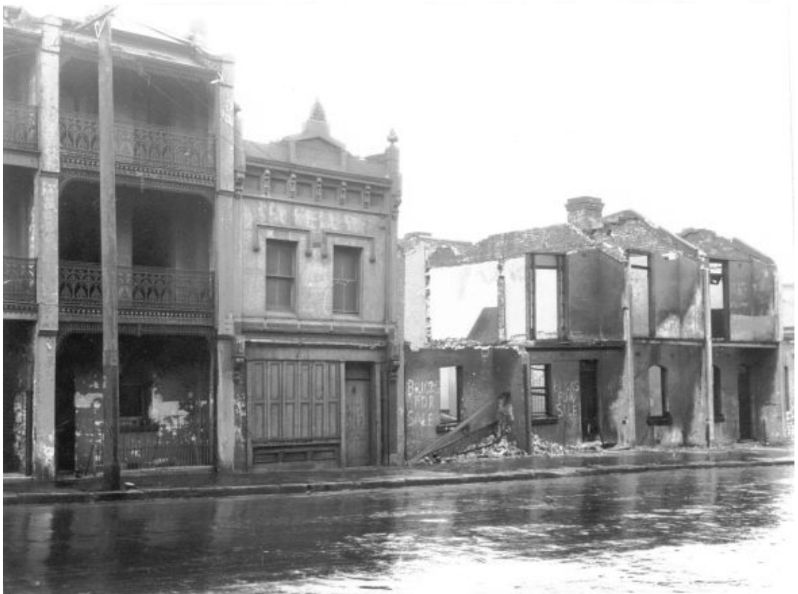
Figure 7-13 October 1930, showing the demolition of buildings on the eastern site from Union Street
