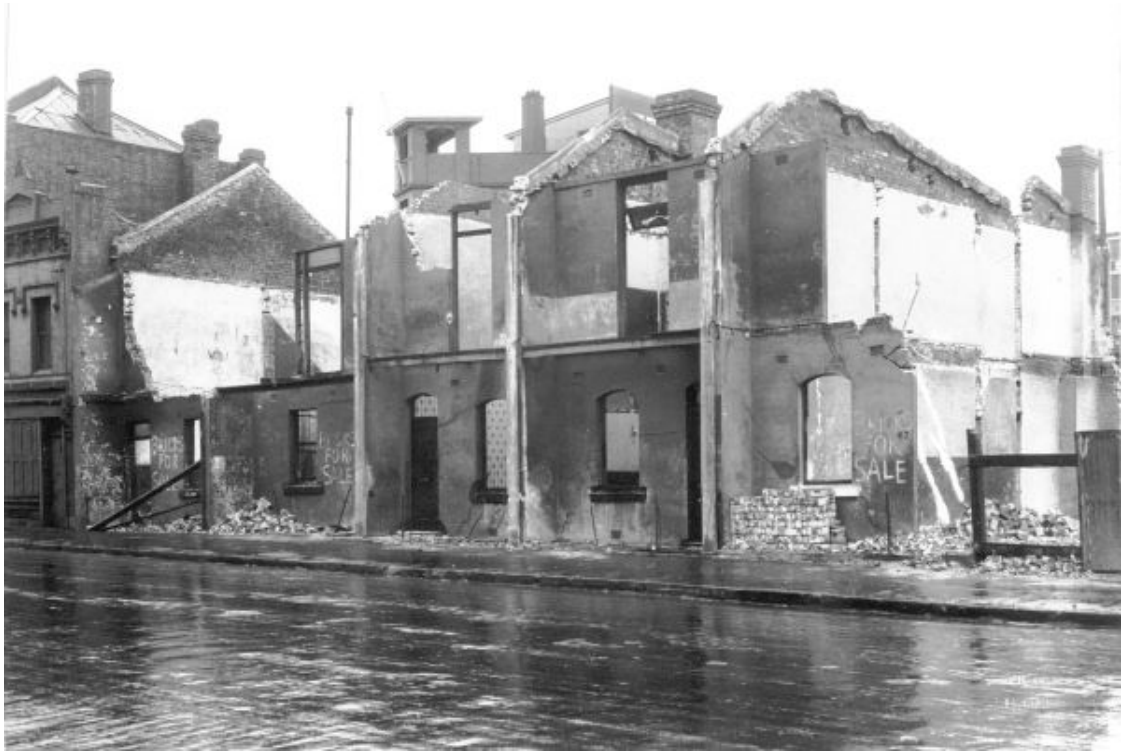
Figure 7-12 October 1930, showing the demolition of buildings on the eastern site from Union Street
