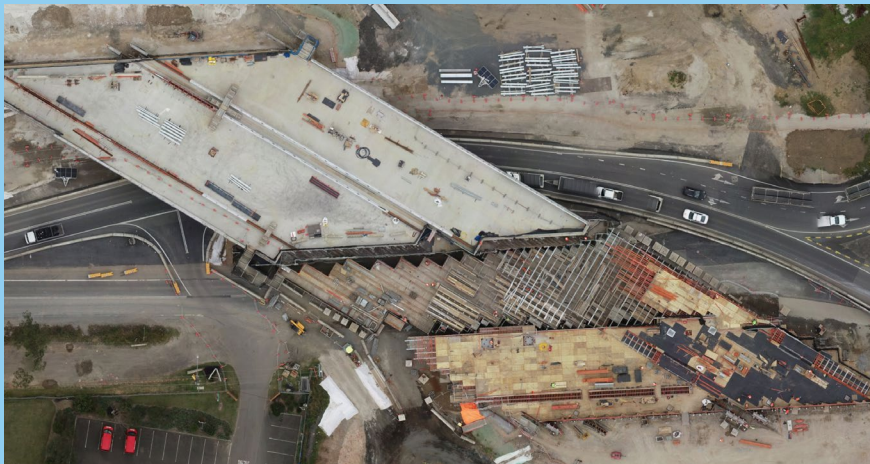
Aerial view of the Elizabeth Drive bridge in Kemps Creek under construction
