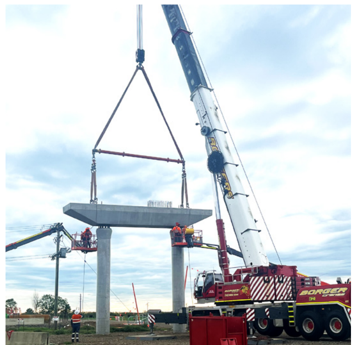
First headstock arriving on site for the bridge over the Doughboy Hollow floodplain
