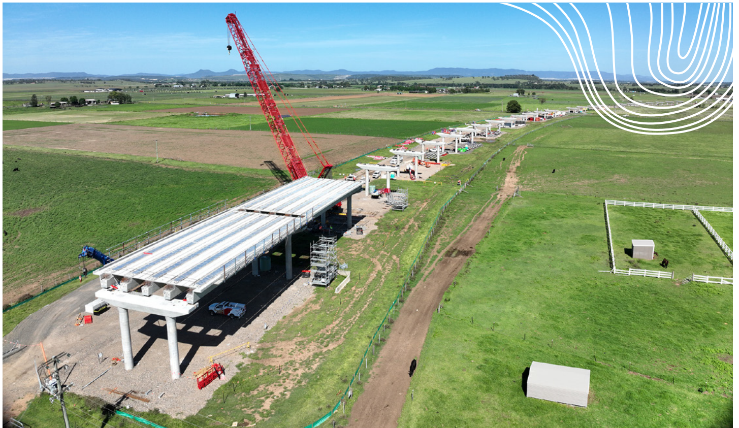
First girders on Doughboy Hollow floodplain bridge, looking towards Army Camp Road
