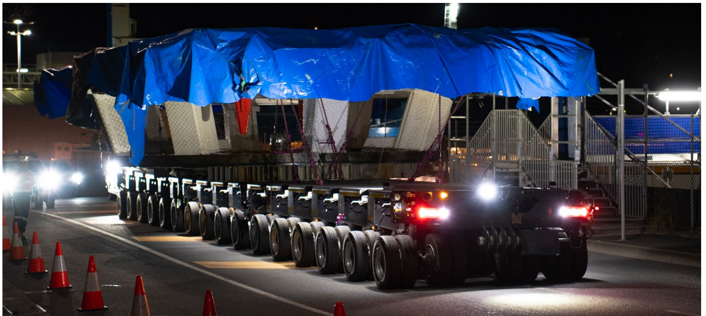
The first TBM part being delivered from Glebe Island across City West Link and into the WHT portals.
