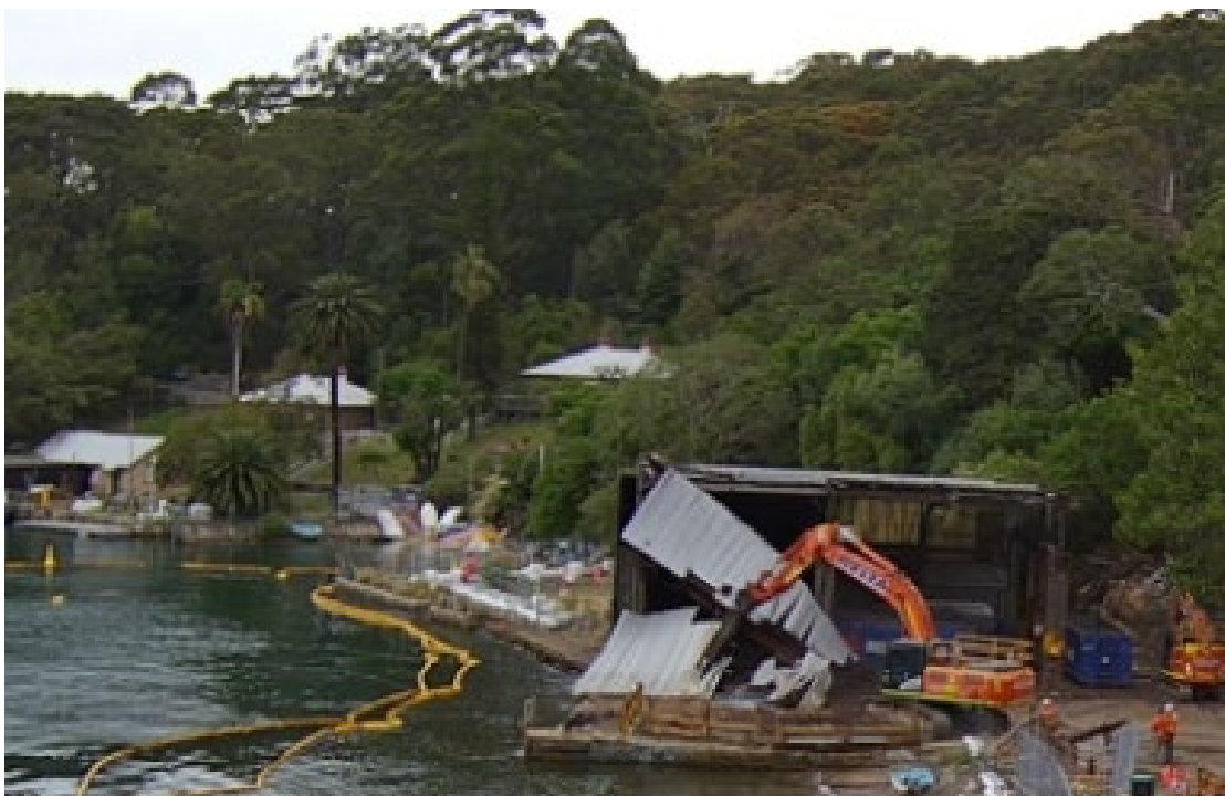
Derelict building demolition, now complete. (Looking south at the former shipyard main building following salvage work).
