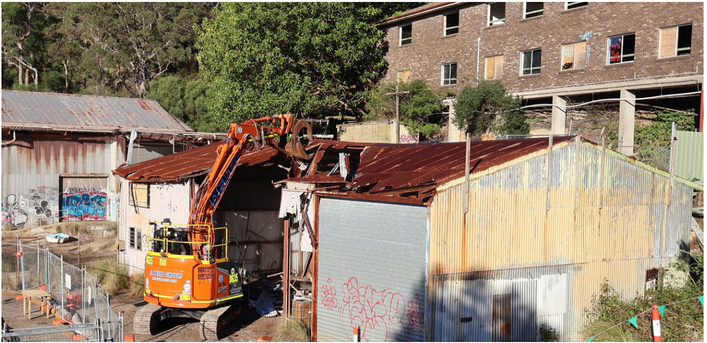
Derelict building demolition, now complete. (Looking south-west at the former workshops and administration building).
