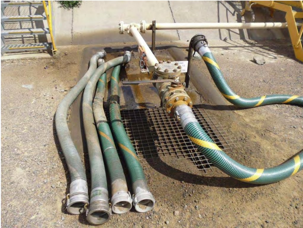
Photo 10 - At the bulk fuel depot, sumps designed to retain any spilled diesel were almost completely blocked with sediment.
