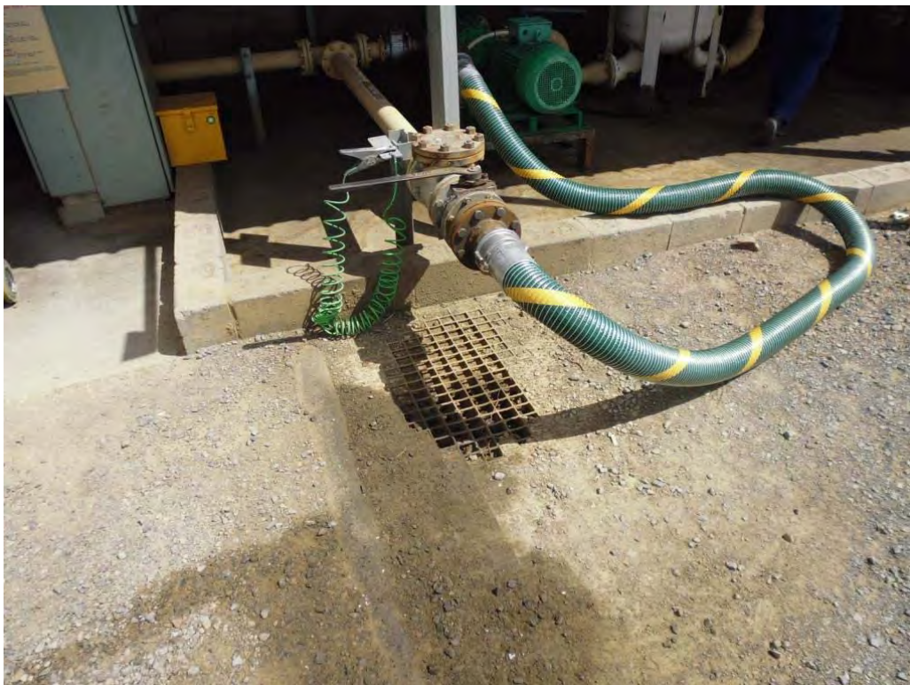
Photo 11 - At the bulk fuel depot, sumps designed to retain any spilled diesel were almost completely blocked with sediment
