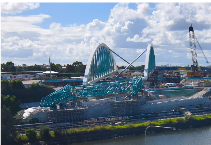
The steel launch nose temporarily attached to the front of the Twin Arch Bridge to facilitate the launch.
