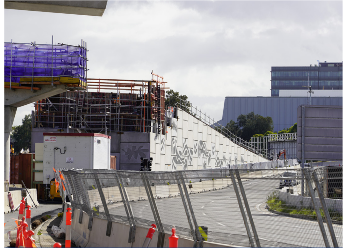
The start of the Flyover ramp continuing to take shape in the middle of Qantas Drive, Mascot.
