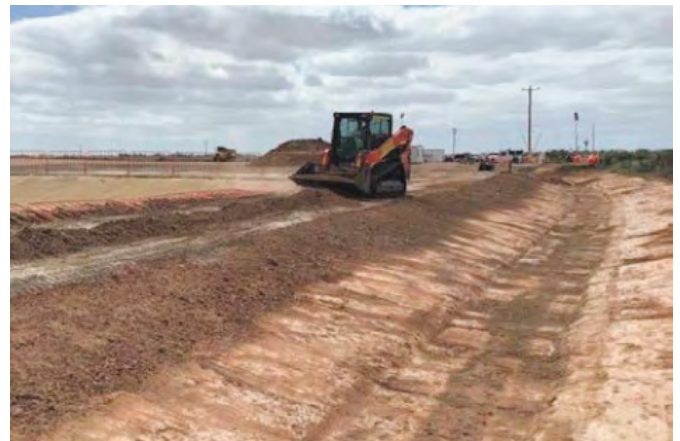
Picture: Swale drain being built to manage water flow on the EnergyConnect project.
