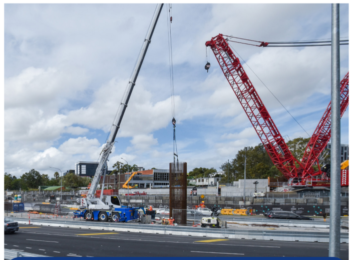
Piling work for piers that will support the flyover on Qantas Drive, west of Robey Street.
