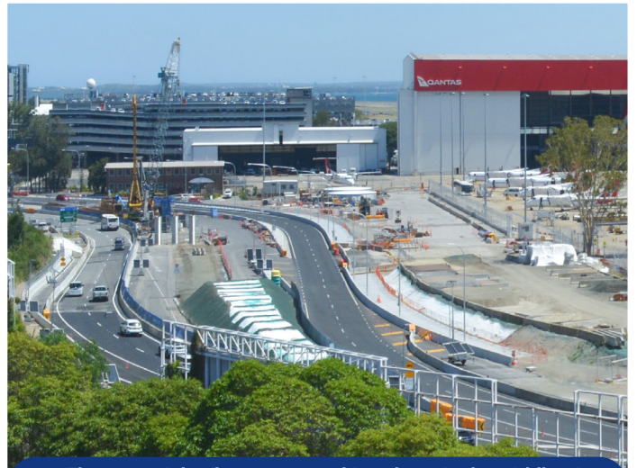
The start of the flyover ramp taking shape in the middle of Qantas Drive, Mascot.
