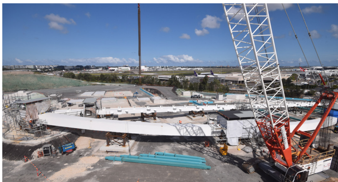
Deliveries have started to arrive at our Tempe site for the twin arch bridges.
