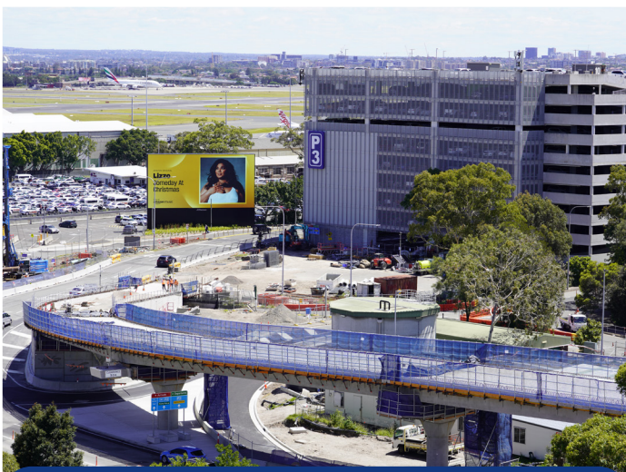
Work continuing on the Departures ramp over Sir Reginald Ansett Drive, Mascot.
