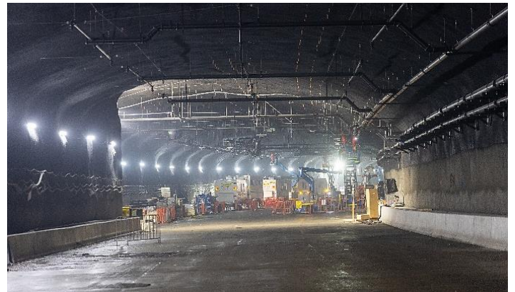
Image: Electrical service installation progress, as well as pavement and barriers shown at Arncliffe, November 2024
